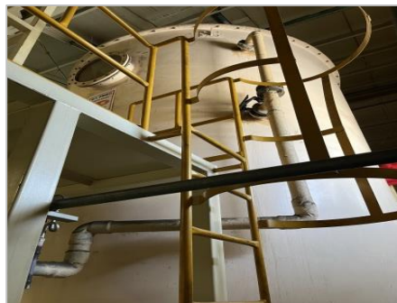
[Scrubbers in the Eonhaa Factory]
